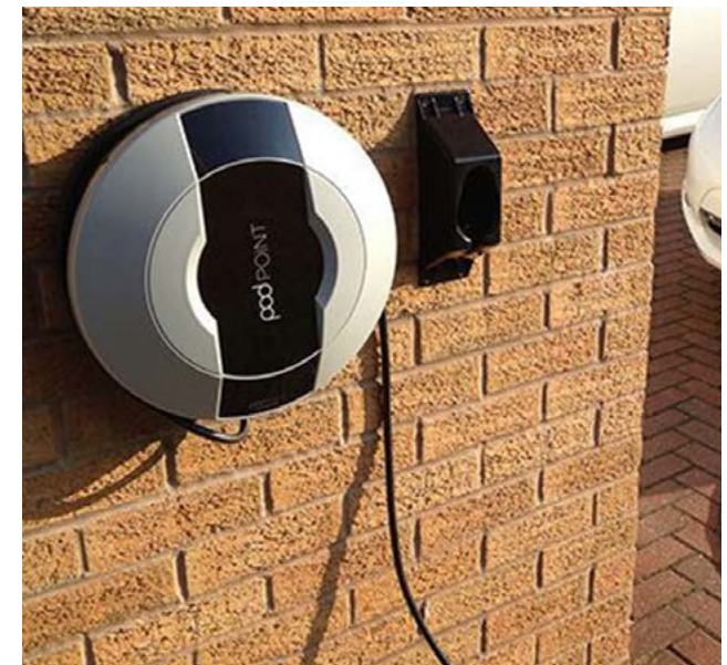
Figure 294: Home electric vehicle charging point.
