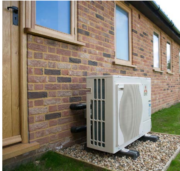
Figure 295: Air source heat pump unit.
